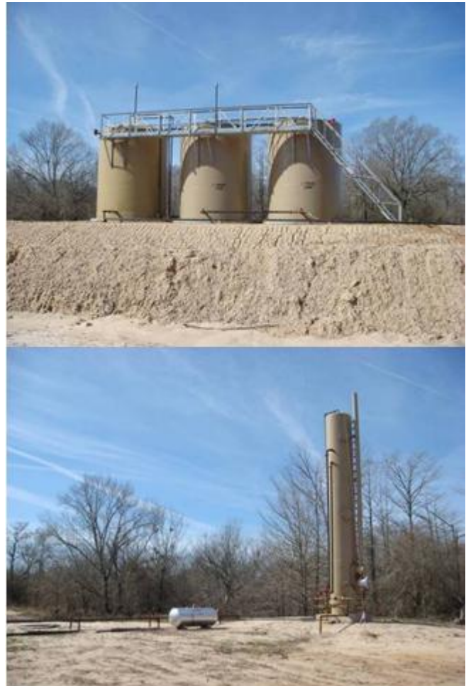
Production Facilities in place at the Saline Point Project, LaSalle Parish Louisiana
