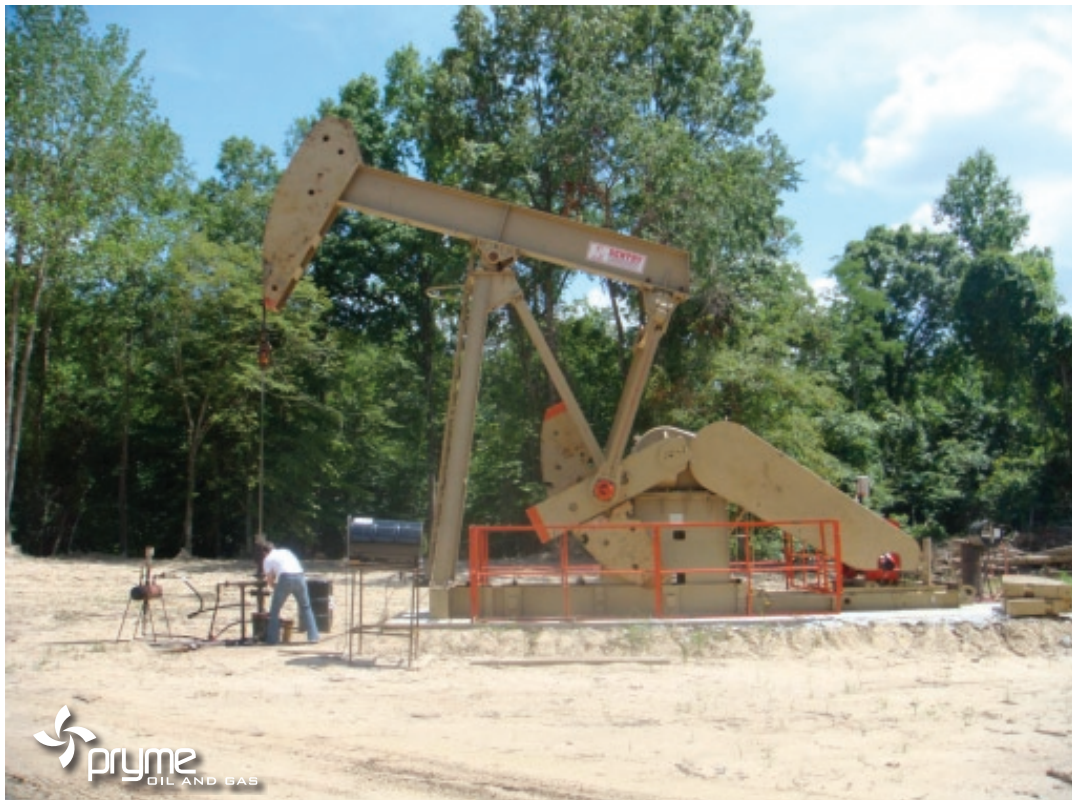
Pumping Unit at the Hall No.1 Well in the Sunny Side Prospect, Four Rivers Project
