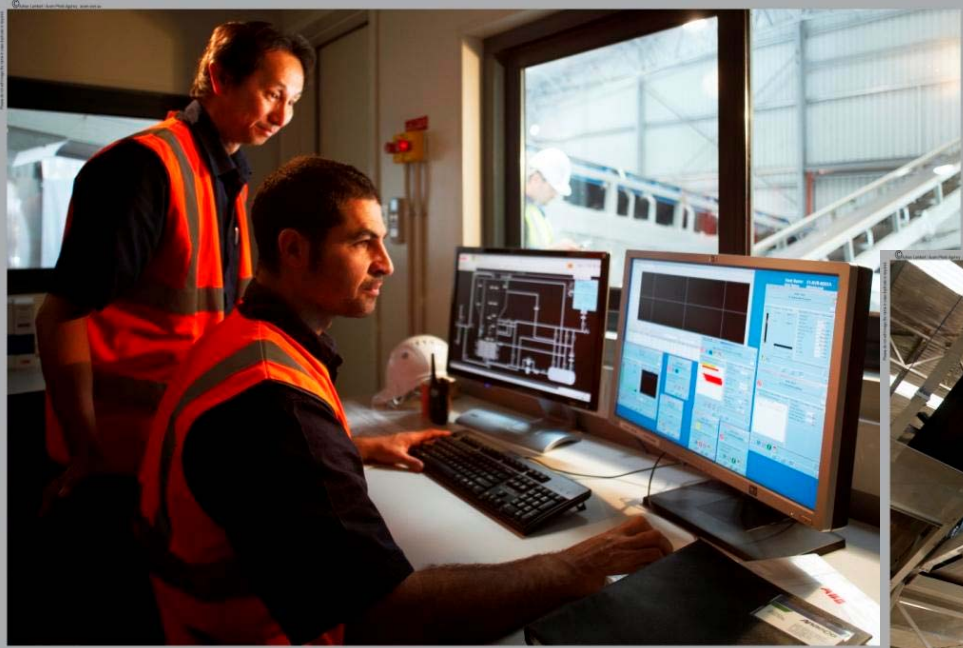
Distributed Control System (DCS) providing the DiCOM System automated operation
