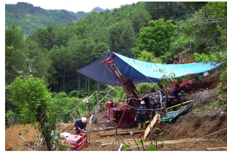
Above: Maxi-195 man-portable drilling inclined diamond hole TRDD004 on West Sentul Vein
