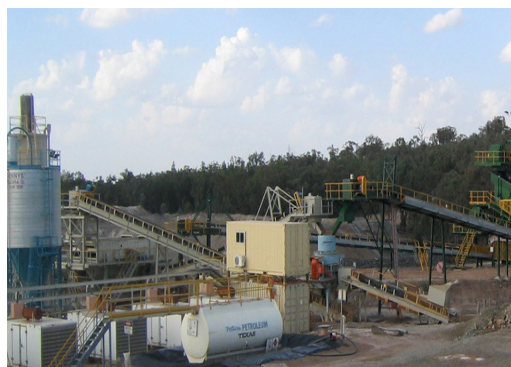
Figure 1 - Plant infrastructure at Twin Hills mine
