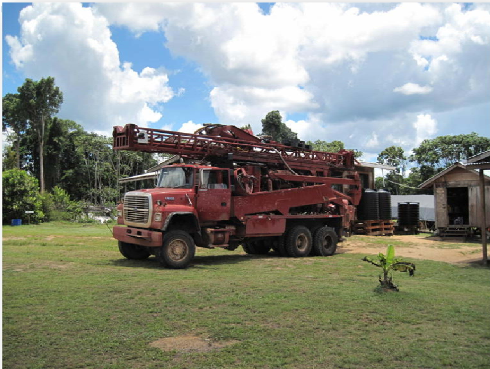
Images of the truck mounted Drilltech D-12 truck mounted rig and support equipment, at the Hicks base camp West Omai Project, Guyana.
