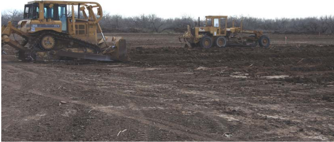
Bulldozers and Graders preparing the Frances Dilworth No. 3H well location for receipt of Nabors Rig M34 in mid-February.
