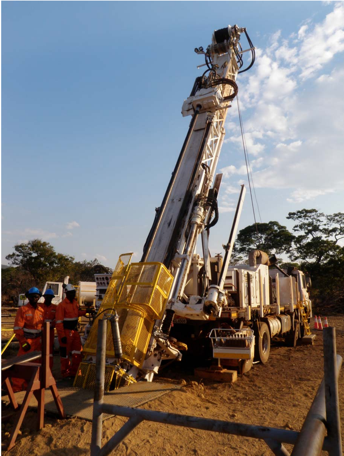
FIGURE 2 – Drilling rig set up over the first hole being drilled at the Mushingashi Anomaly.
