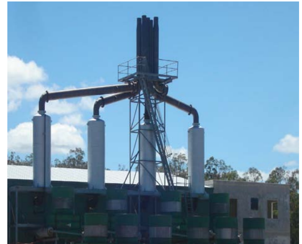
External equipment in place - January
