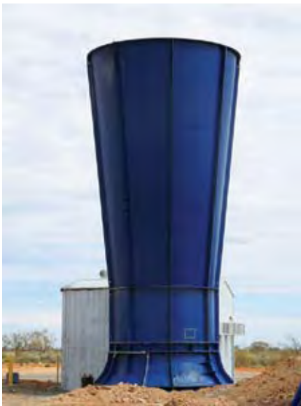
Surface fan over the ventilation shaft
