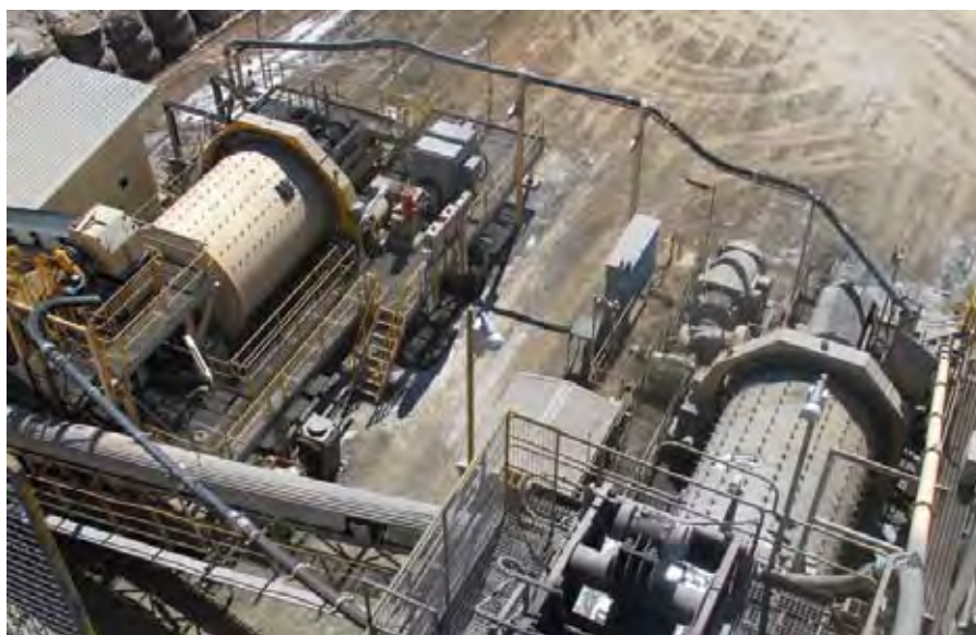
The second ball mill in series with the existing mill
