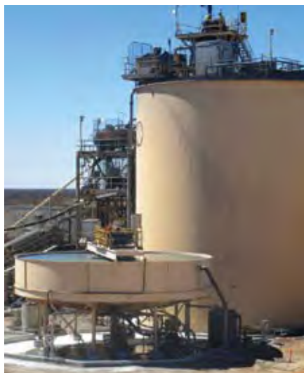
Thickener with upgraded cyclone tower and control room
