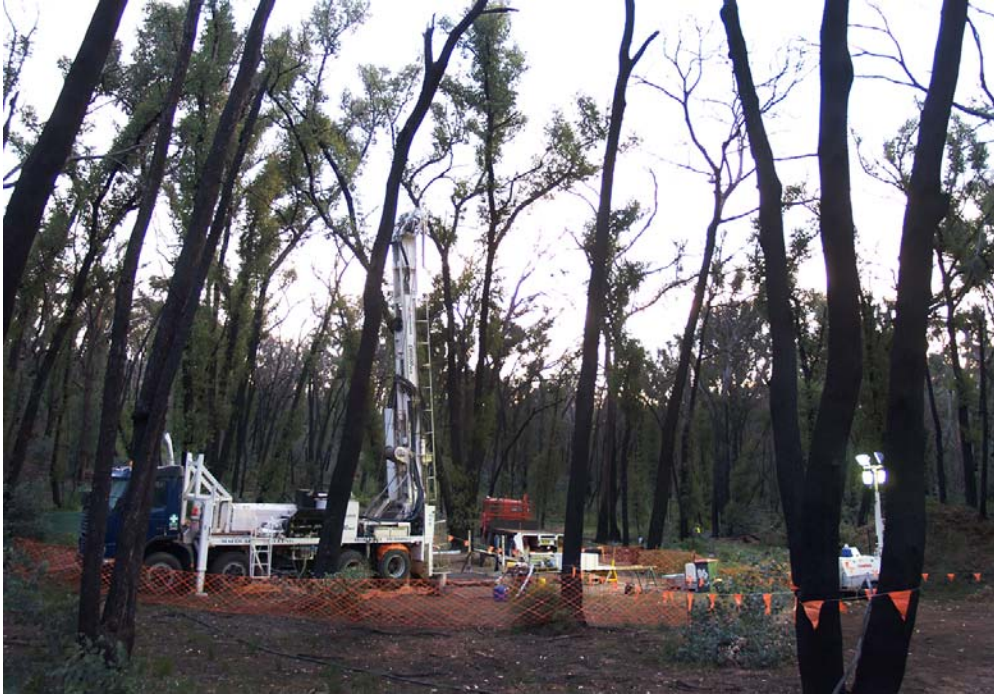
Night Shift Diamond drilling in progress at Belltopper Hill – Malmsbury Gold Project
