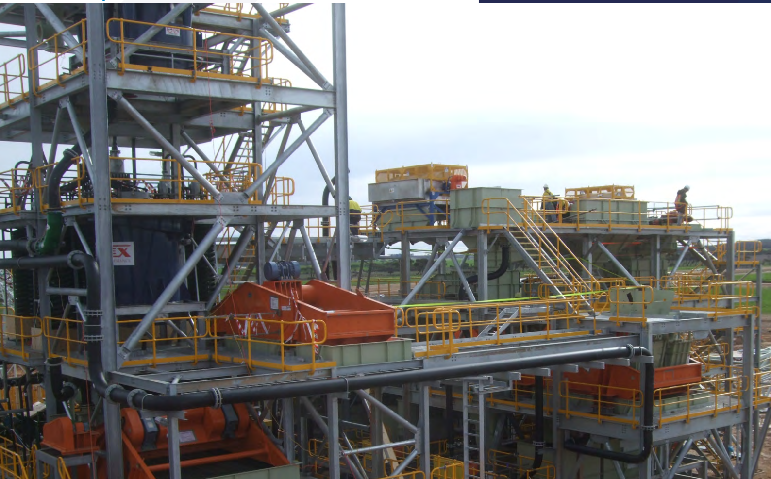
Mt Cattlin Heavy Media Plant
