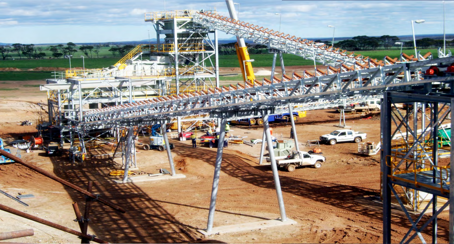
Mt Cattlin Crusher Plant
