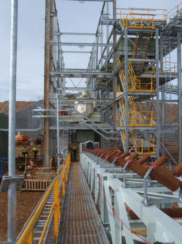
Mt Cattlin Crushing Plant
