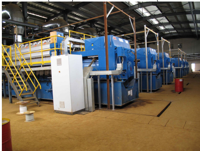
Power Station (30 MW) at Kurumbukari Mine Site (Ramu Nickel-Cobalt Mine).
