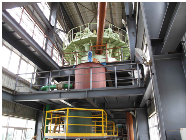
Cyclones at Beneficiation Plant at Kurumbukari Mine Site (Ramu Nickel-Cobalt Mine).
