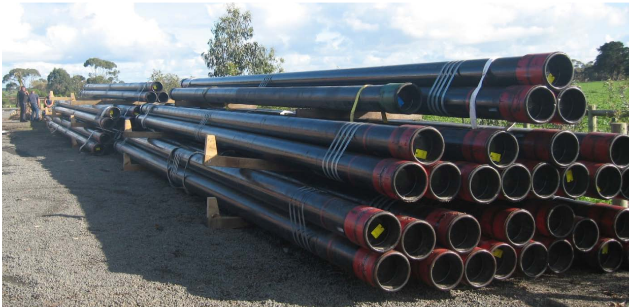
Figure 4: Part of the 9-5/8 inch production casing order for well KHR-1 stacked at Koroit storage facility, ready for commencement of proof of concept drilling
