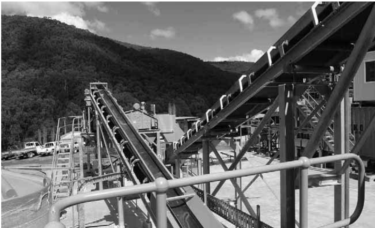
View of undersize/oversize conveyors on the new GPP's crushing circuit
