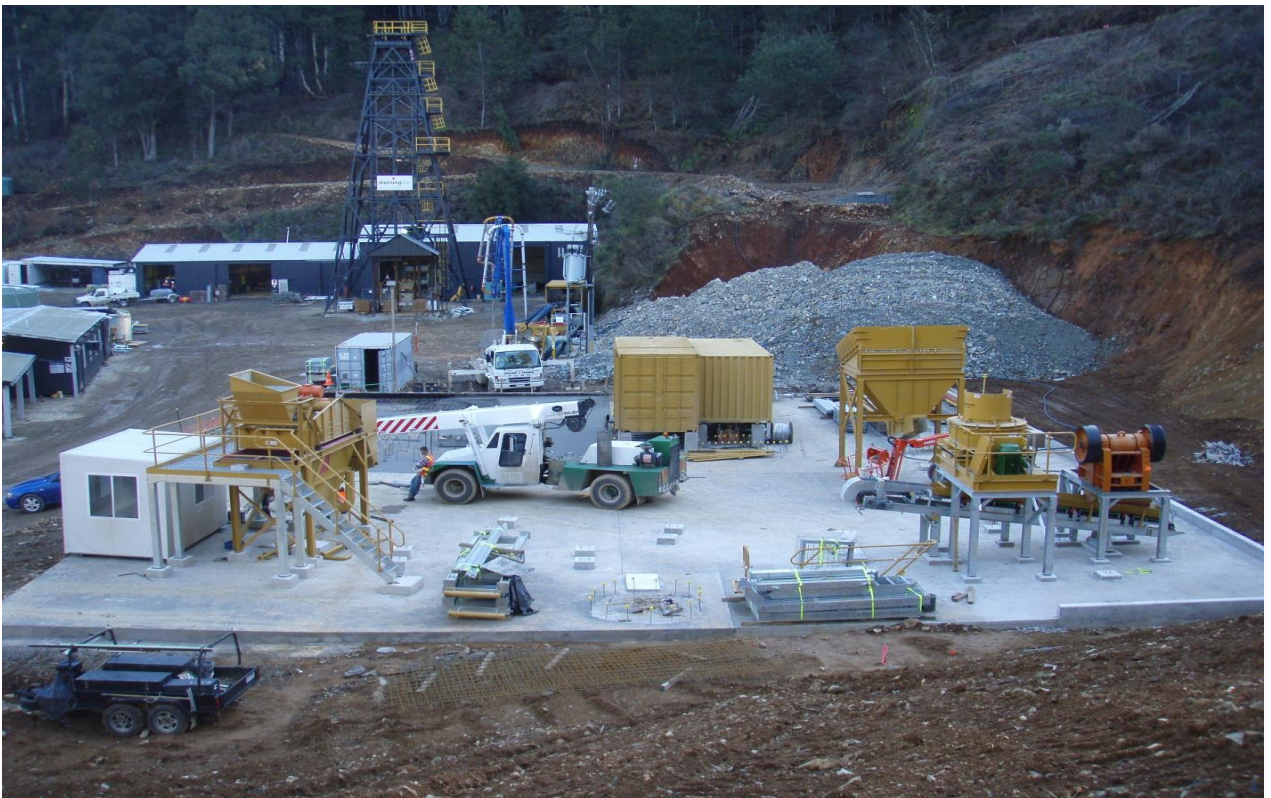
MCO's onsite Gravity Processing Plant (GPP) under construction during the Sept. Quarter 2010
