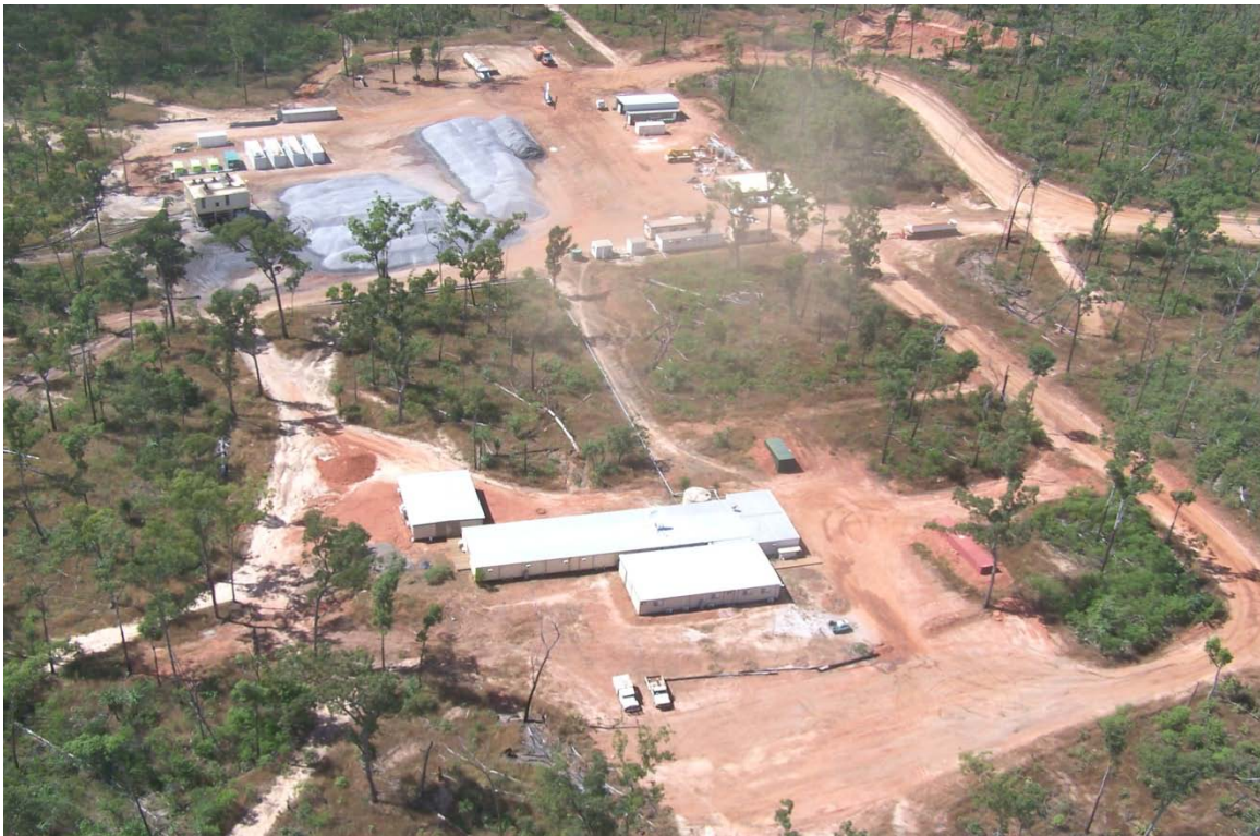
Andranangoo Processing Plant and Camp to be moved to the Lethbridge site in April/May
