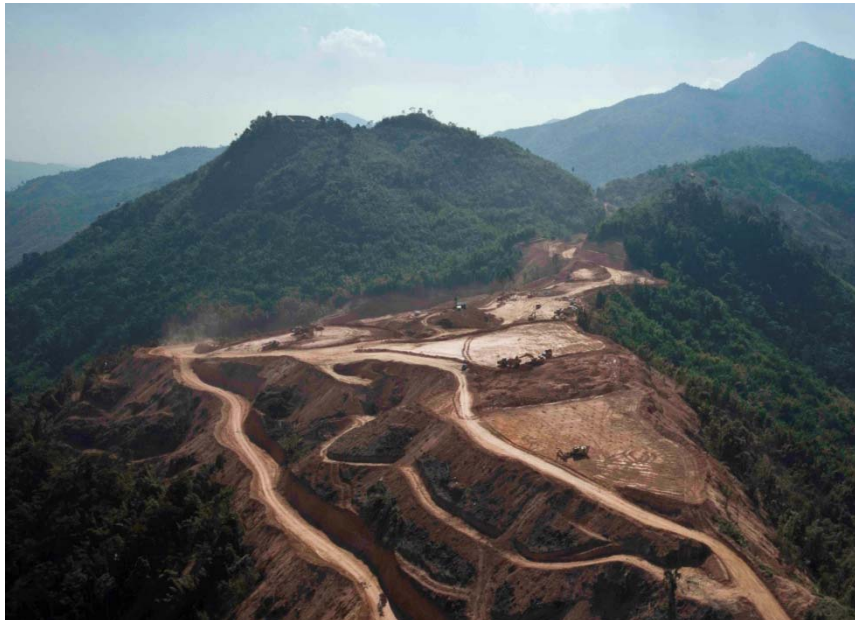
Major earth works at Ban Houayxai are well advanced; process plant area
