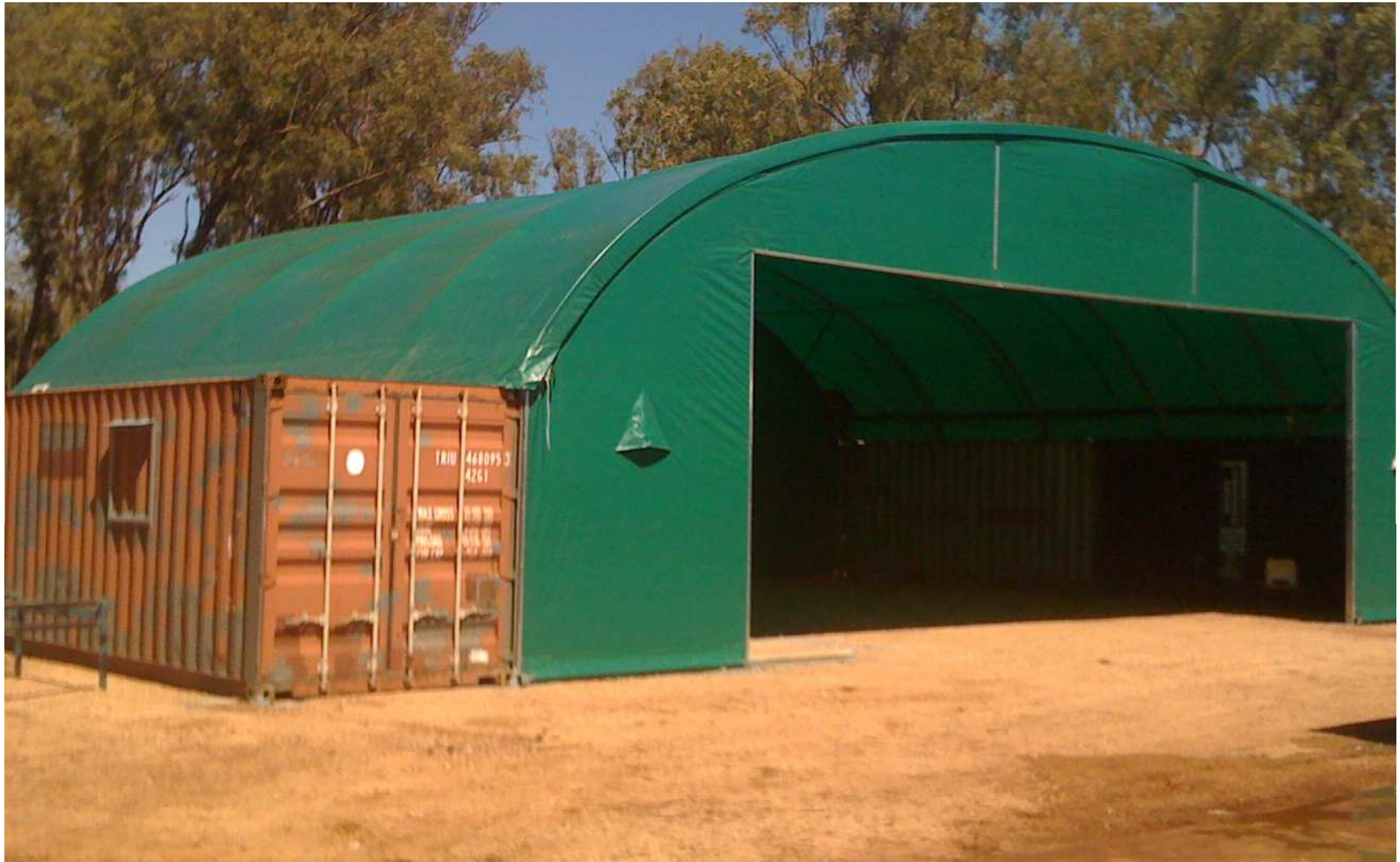
WALKAMIN FACTORY SOUTHERN SIDE WORKSHOP, CLIMATE CONTROLLED PRODUCT STORAGE AND PLANT STORAGE WORK INPROGRESS
