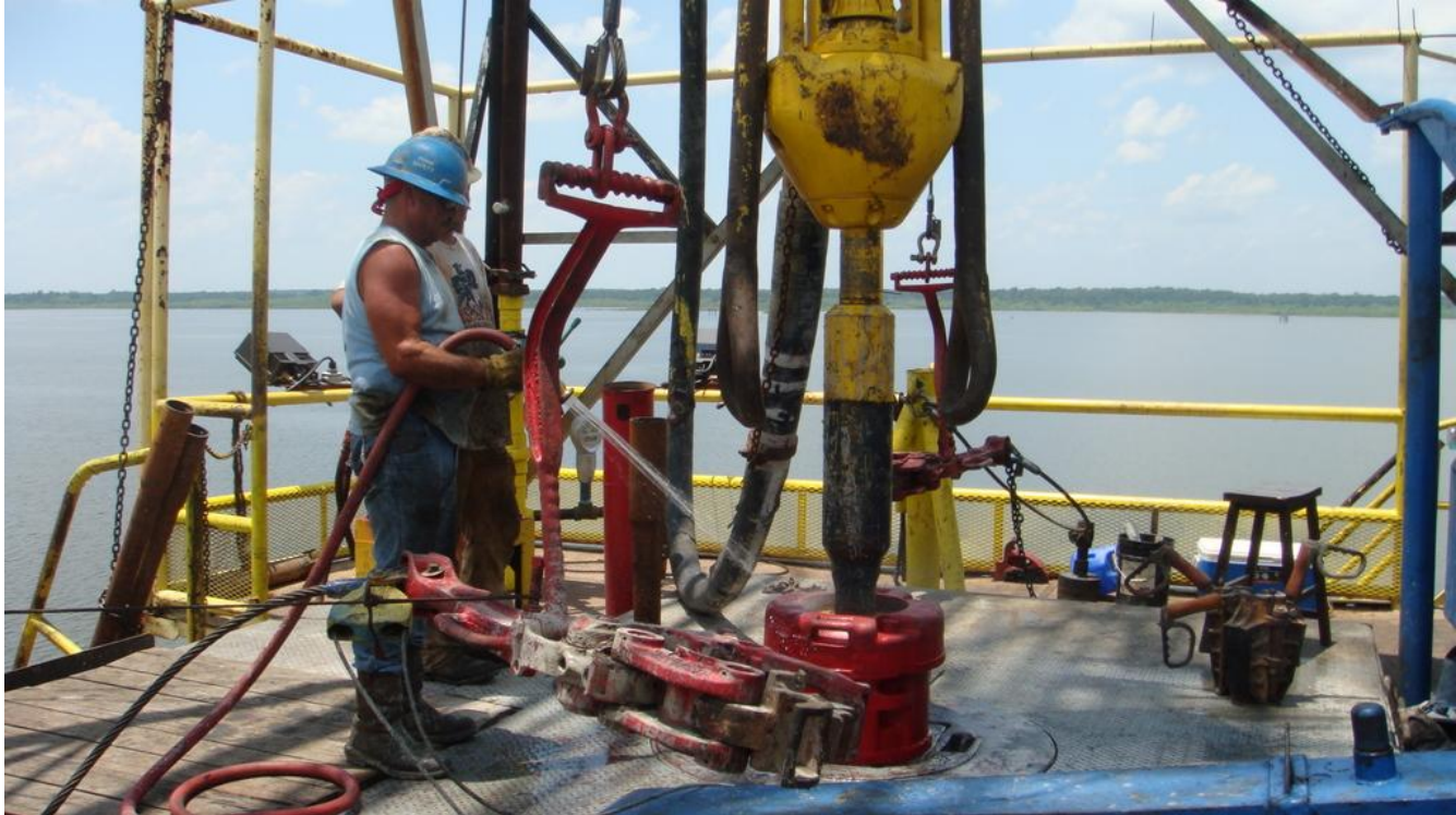
Drilling crews working on the barge mounted rig in Catahoula Lake, Louisiana
