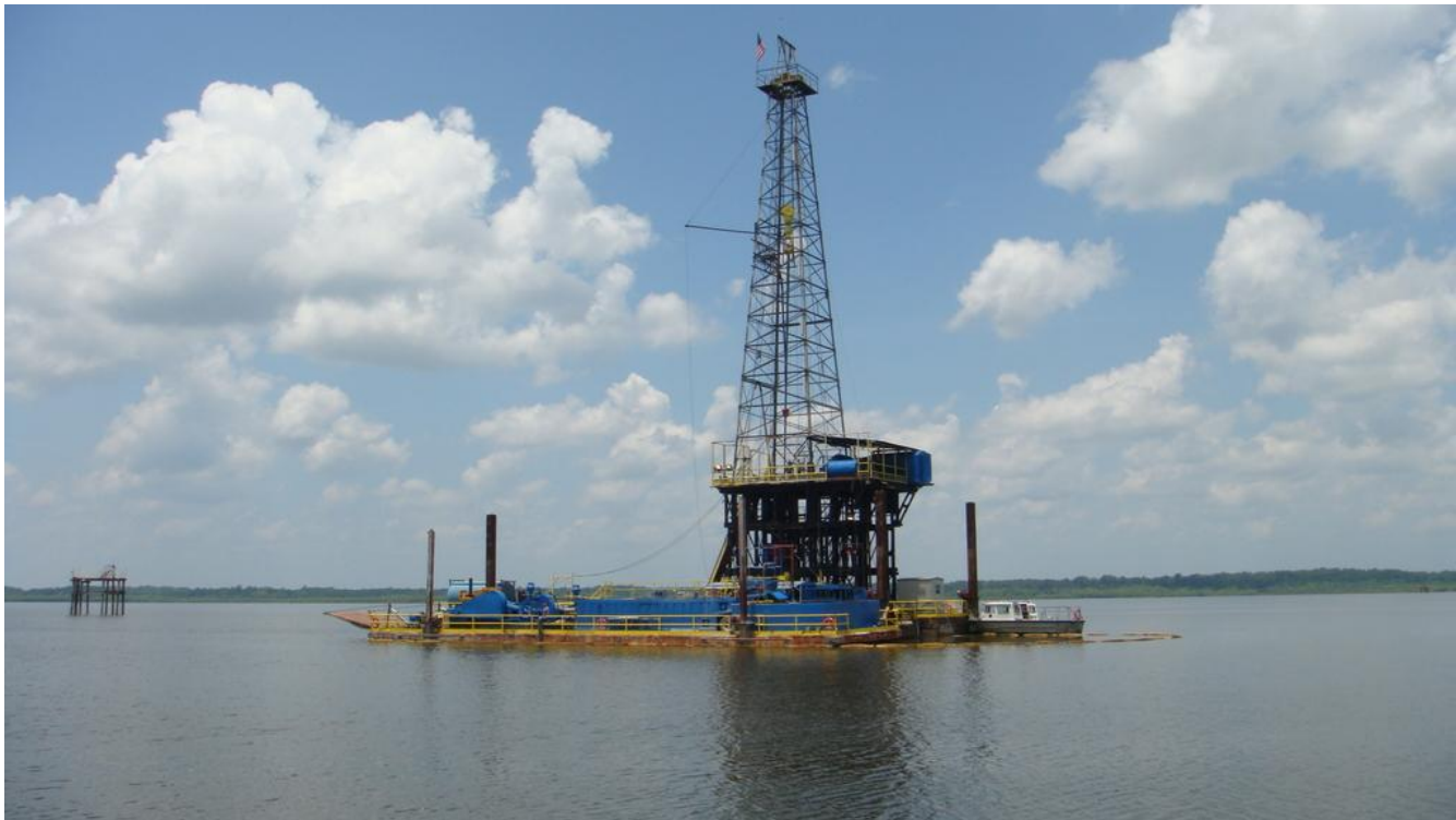
Drilling of the SL 502 No.1 from the newly refurbished barge mounted rig in Catahoula Lake, Louisiana
