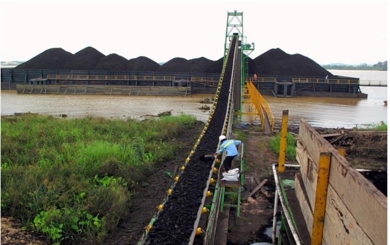
Figure 4 – Current conveyor loading operations for NAD.
