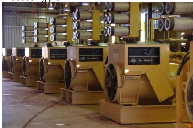
Power station generators
