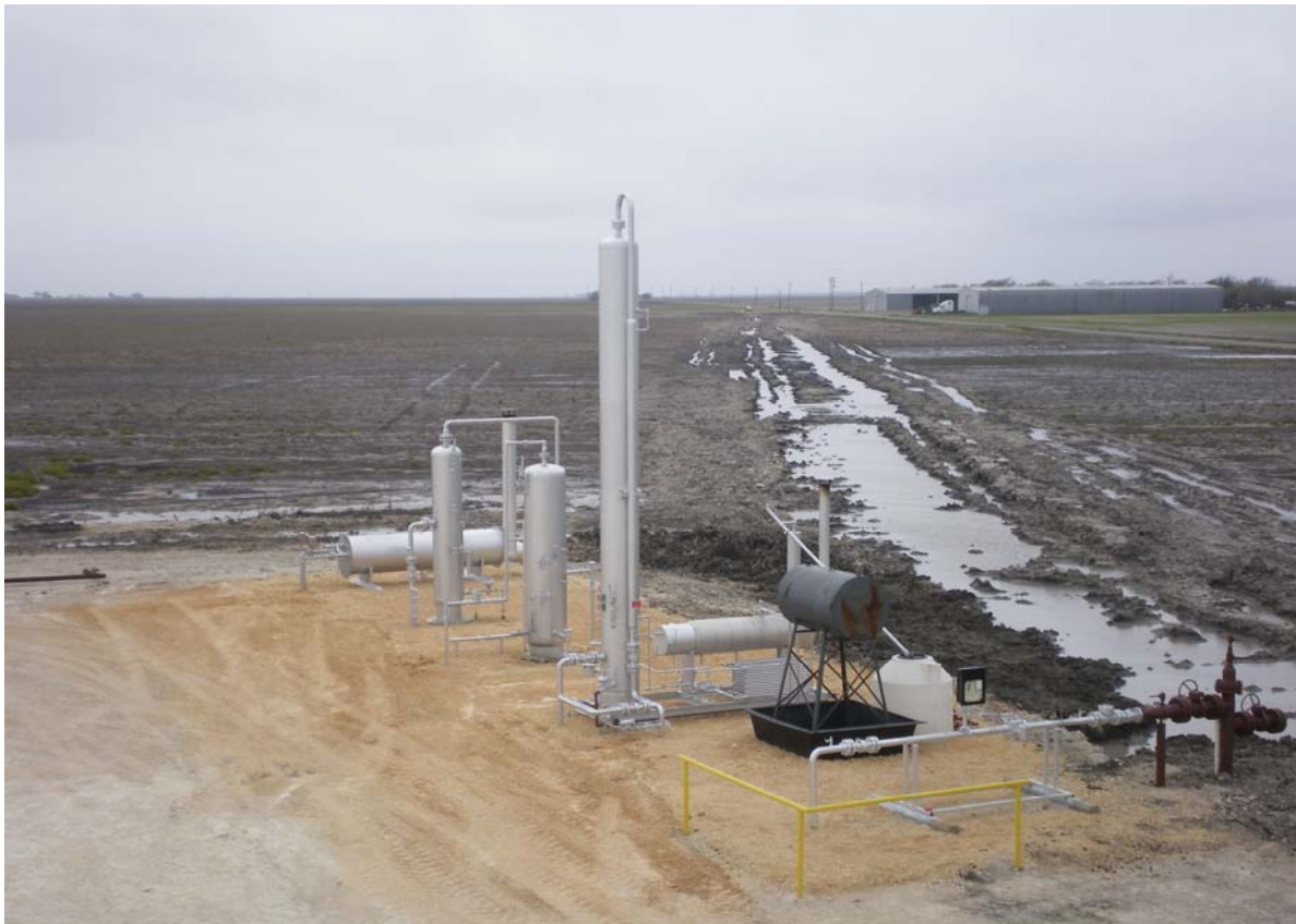
Figure 1 – processing facilities at the Smith #1 well site
