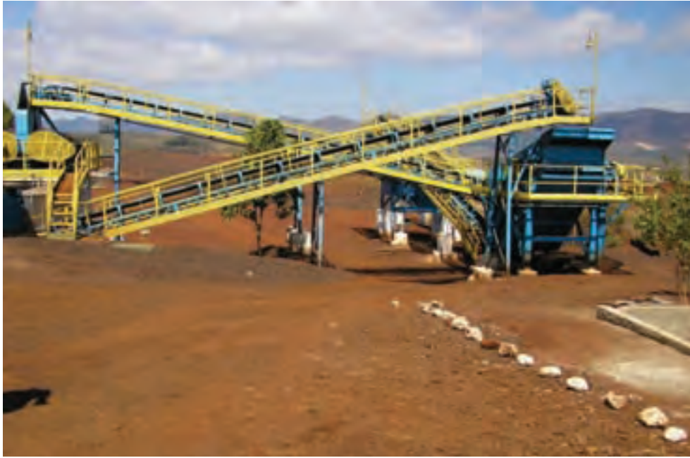
Figure 5.5_1 View across existing Ponto Verde plant
