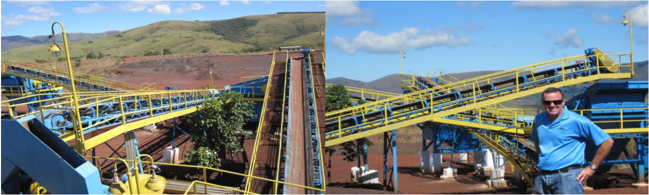
Existing on Site Plant capable of producing 1.8mtpa – No further Capital Expenditure Required
