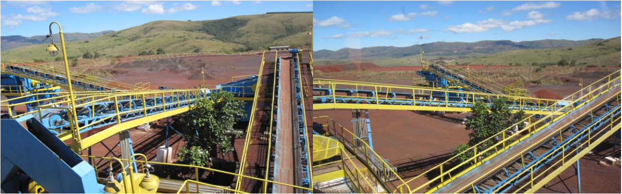
Existing on Site Plant capable of producing 1 million tonnes per annum
