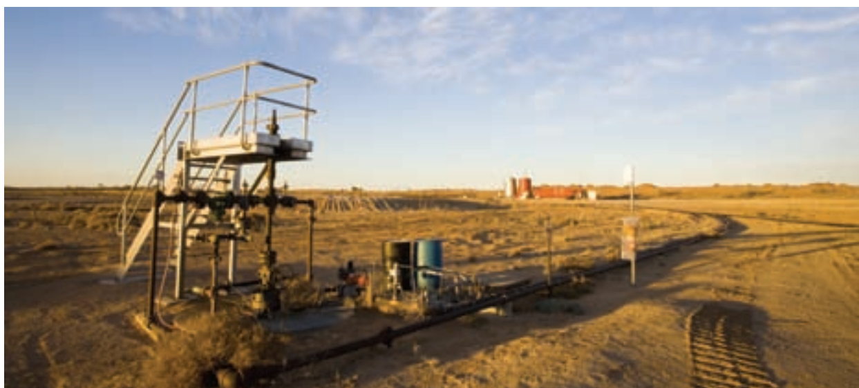
Above: Wireline access platform allowing safe access to the wellhead – Stuart oilfield installation – Cooper Basin
