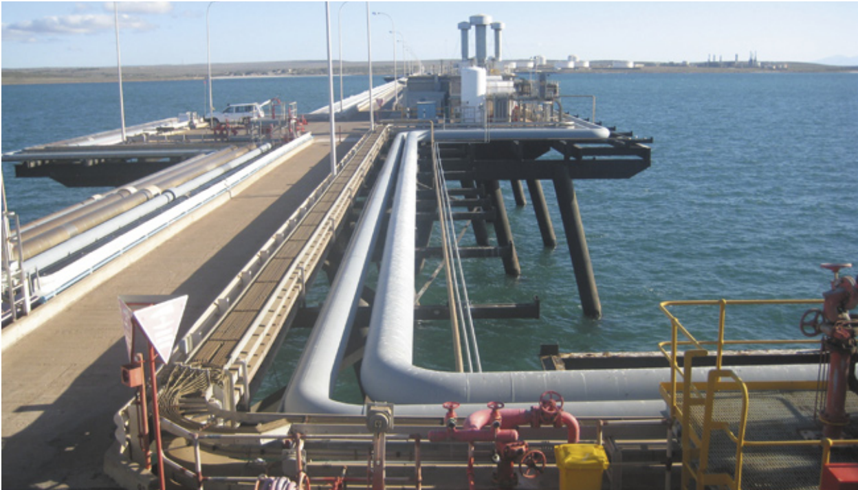
Port Bonython Jetty looking landward towards the facilities which adjoin Stuart's Fuels Terminal site
