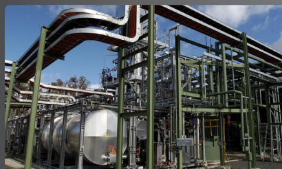
45MLpa Biodiesel production facility in Picton, WA
