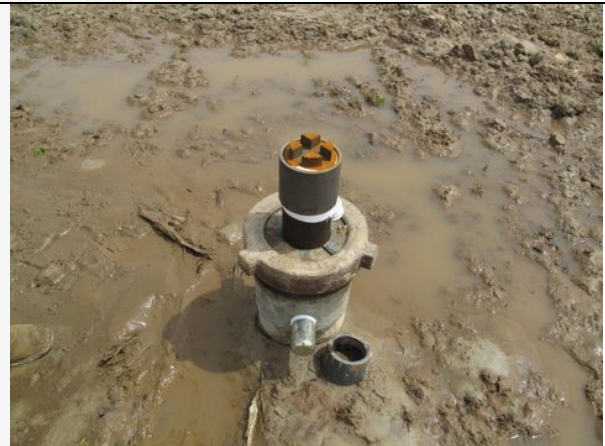
Saltwater Injection Well Wellhead
