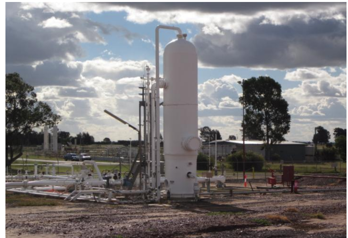
Wallumbilla LPG Plant
