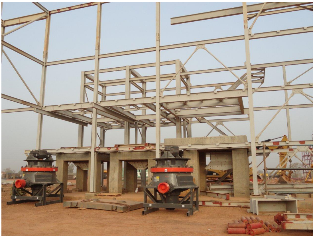
FIGURE 1 - 4 –Construction progress at the Perkoa Zinc Project in Burkina Faso, West Africa
