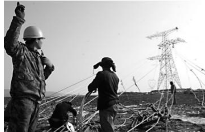
New transmission lines, Mudanjiang: China Daily
