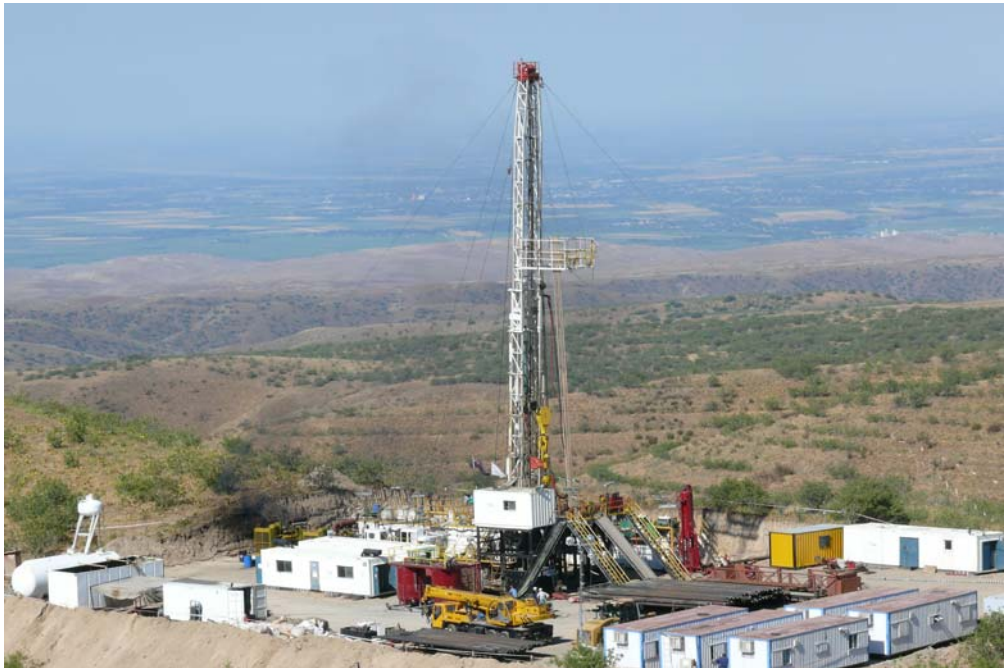
Figure 1- West Mailisu # 2 well site
