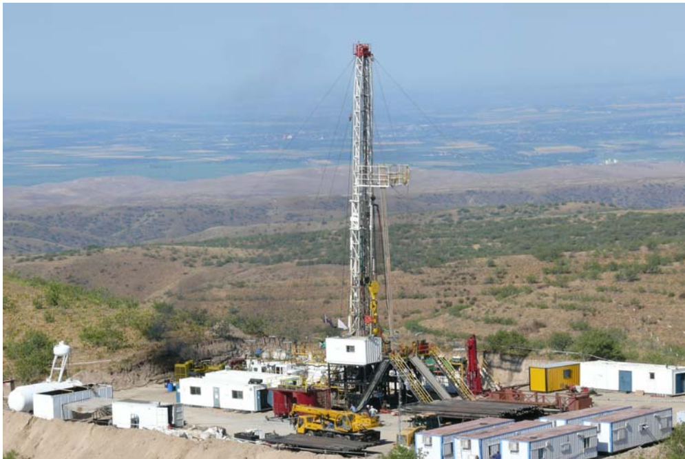
Figure 1- West Mailisu # 2 well site
