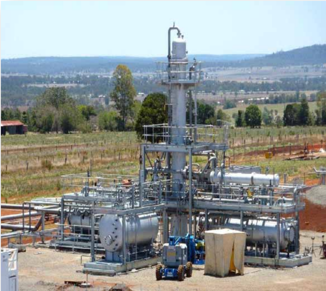
Gas processing plant
