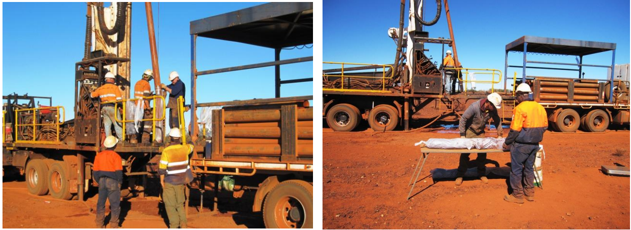
Figure 5 – Photos of Sonic drill rig showing collecting, laying out and measuring large diameter sample
