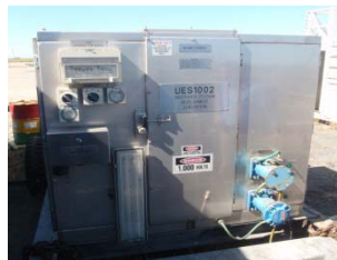
Two Substation – Amprocontrol
