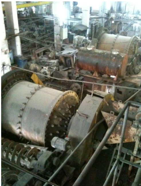
Baita Mill Circuit
