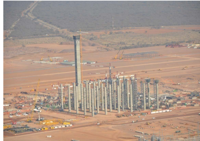
Medupi Power Station
