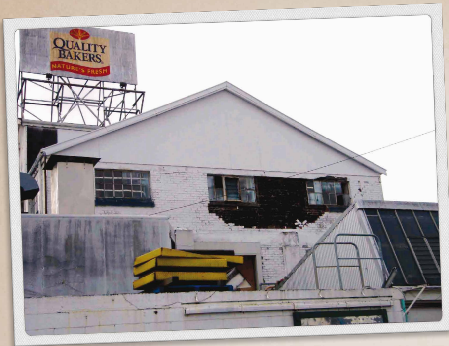
Damage to the Christchurch Quality Bakers site following the earthquakes.
