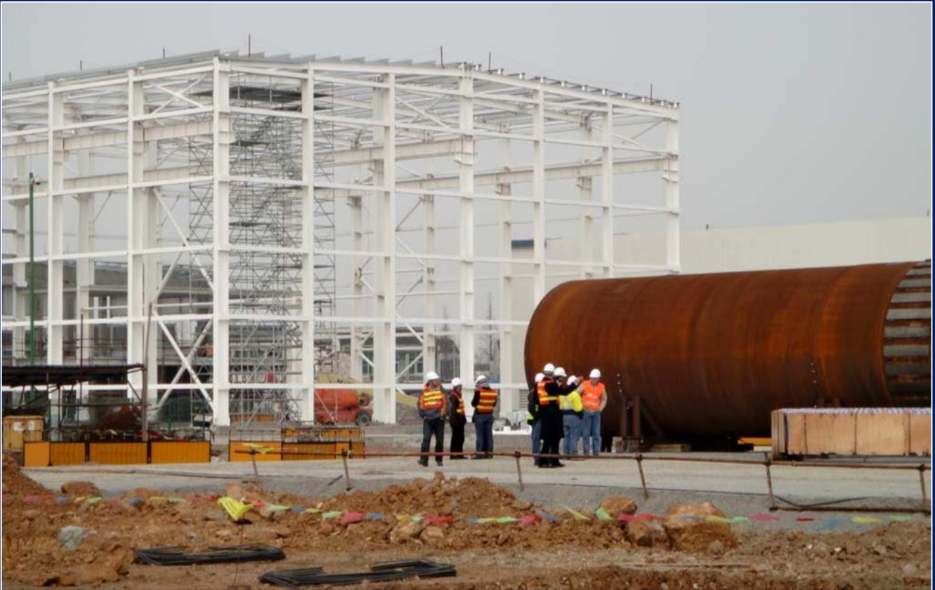
Calcliner kiln shell with processing building in background
