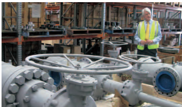
Figure 14: Full inventory of all well head valves and associated equipment for both of the two deep "Proof of Concept" HSA wells have been procured and fabricated and are currently in storage at the manufacturers yard, ready for delivery to Koroit as soon drilling commences.
