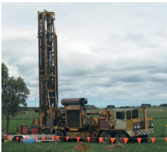
Figure 13: Ground water well drilling operation at Koroit. Drilling water supply for the first deep "Proof of Concept" HSA well, now tested and proven, ready for drilling to commence.
