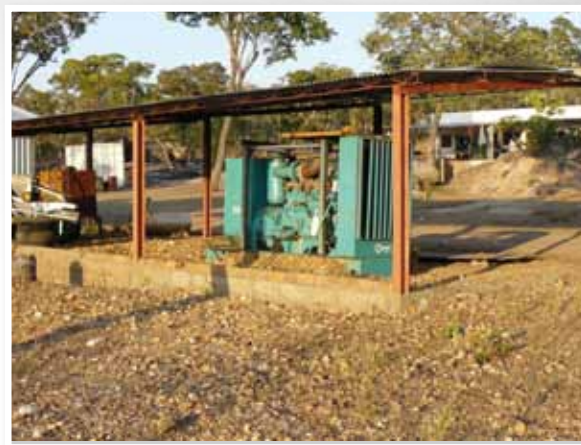
Figure 16 – Site infrastructure in place at GWM's topaz mining operation.
