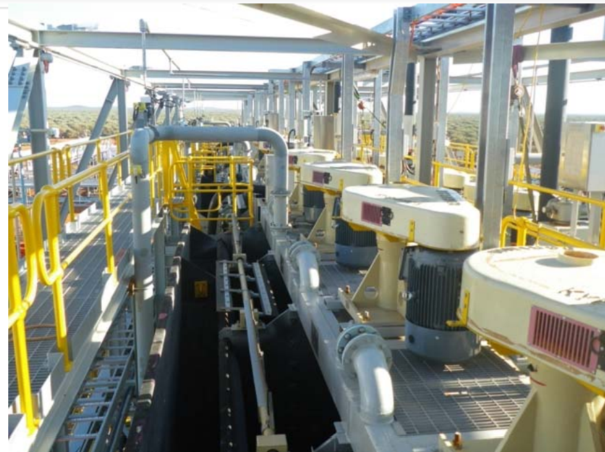
View along top of Flotation Circuit
