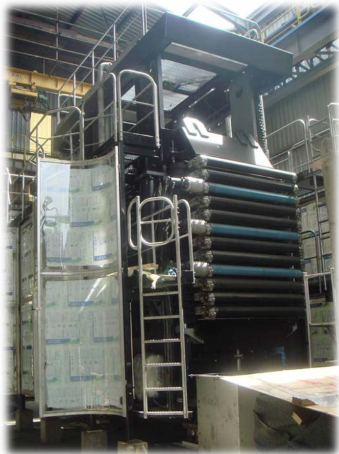
Larox Filter Installed
