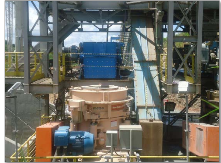
Pebble Crusher Installed & Operating
