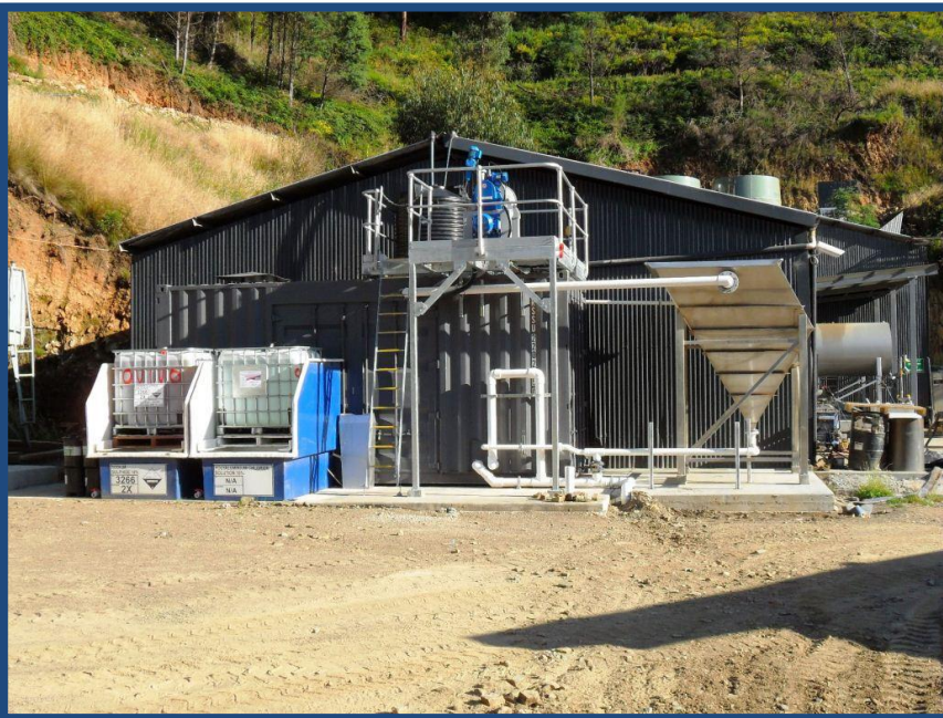
Morning Star's new water treatment plant (As.)
