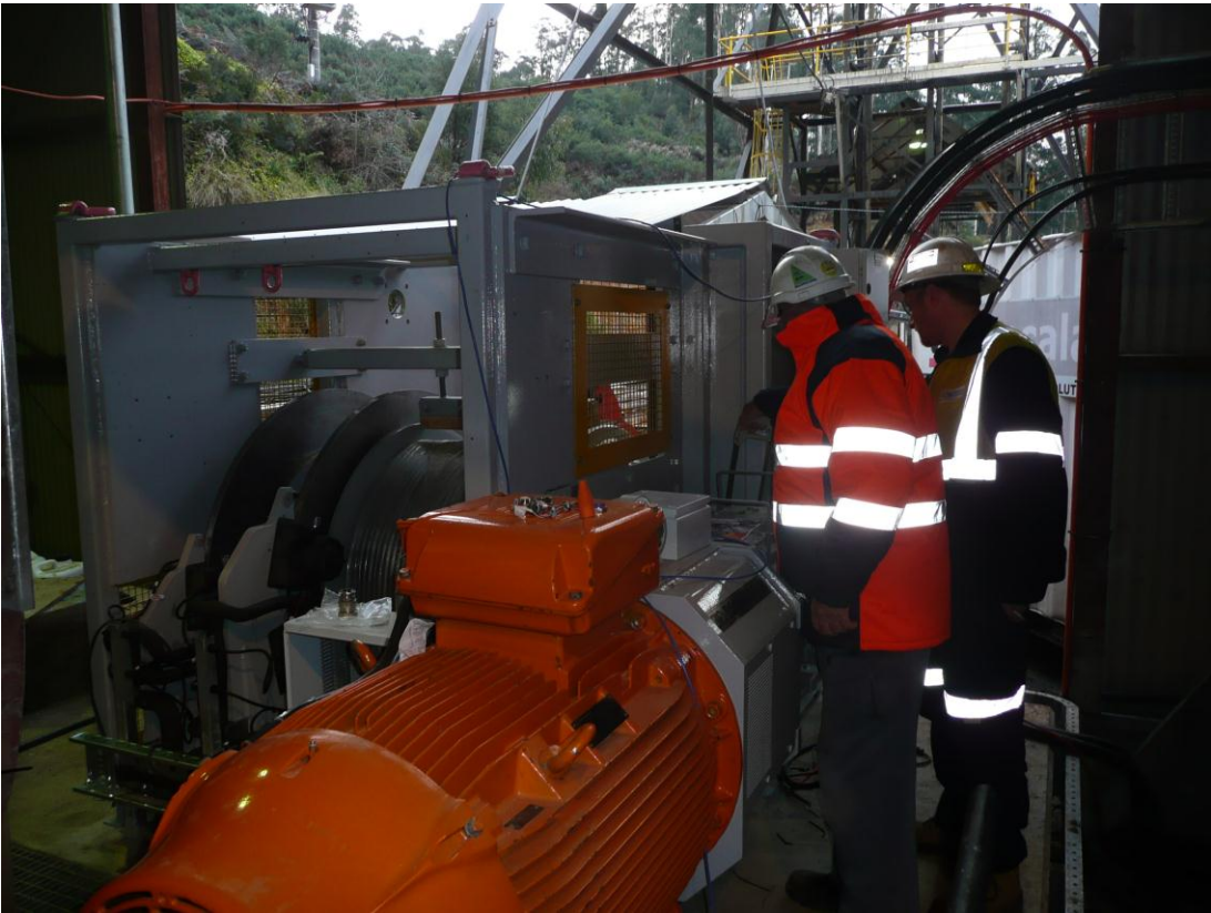
New 160kW Winder at site undergoing final commissioning
