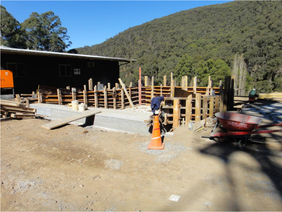
Fabrication of the Overflow Bund for Paste-fill plant at Morning Star Goldmine
