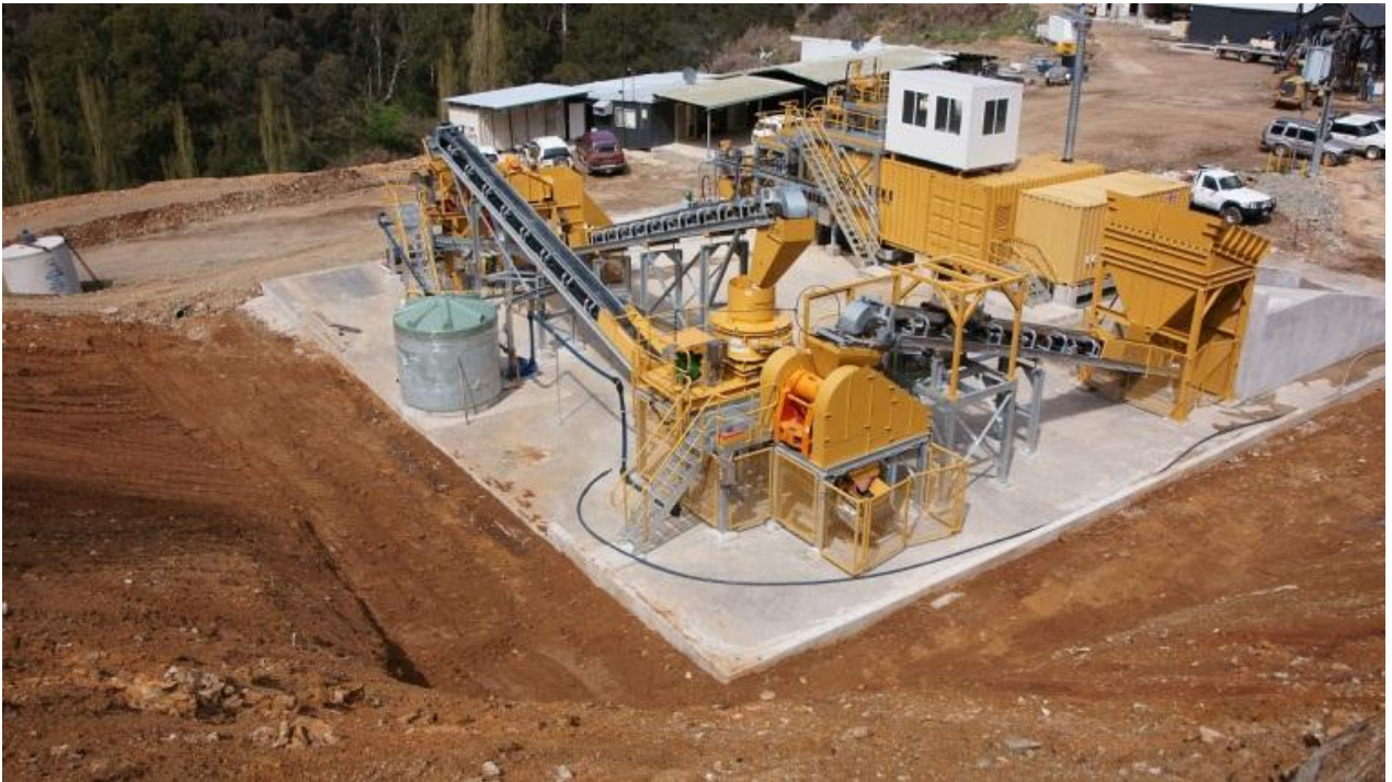
Morning Star's new onsite gravity processing plant (GPP) during the Dec quarter 2010
