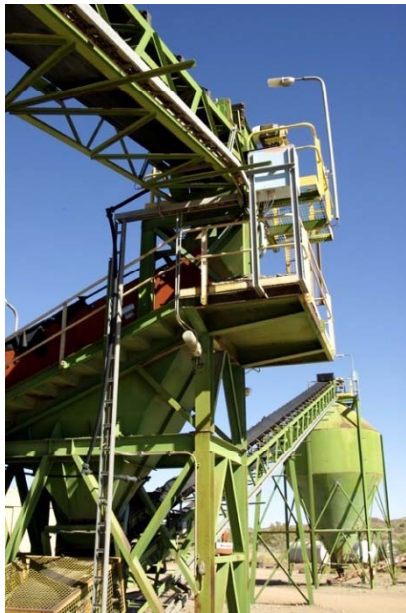
CIP treatment plant on site
